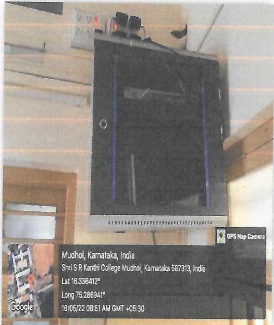
MAIN CONTROLLING HUB
