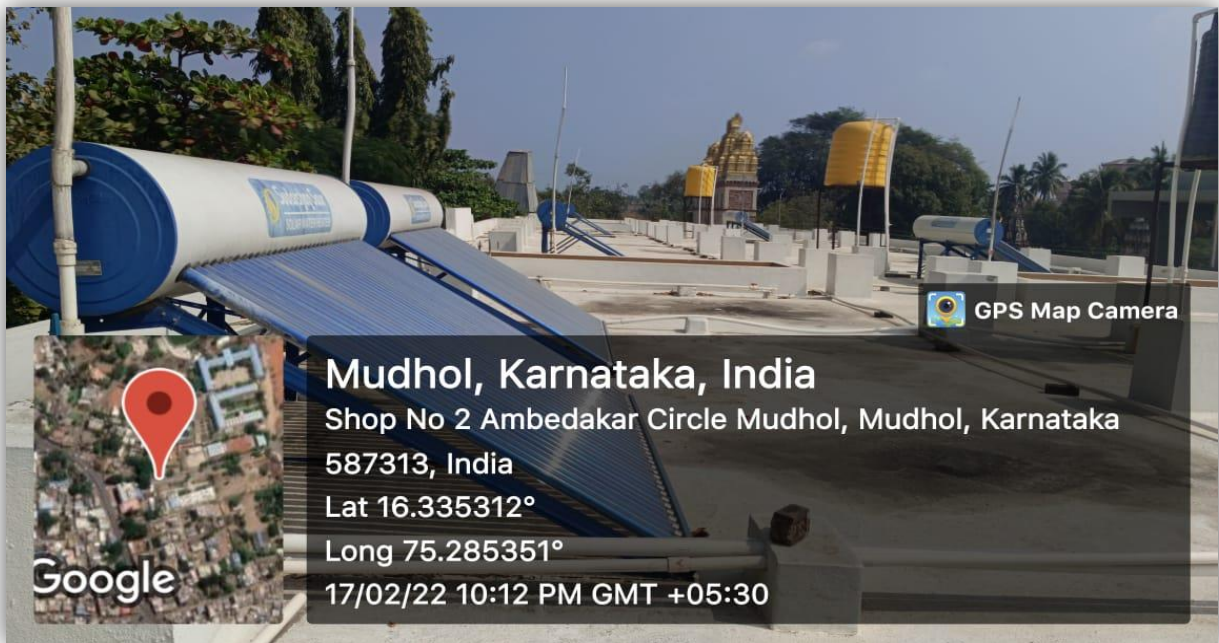
SOLAR PLANT FOR LADIES HOSTEL
